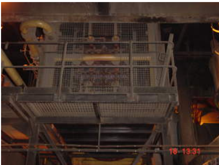
Photo 1: The gas burner installation of the Gluten 20 dryer
